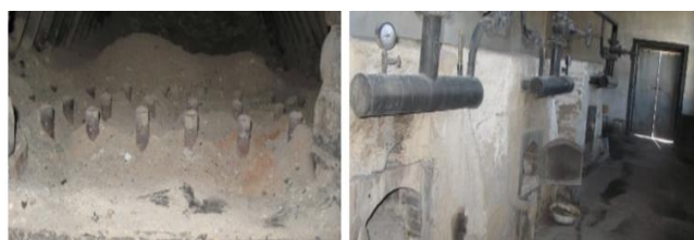
Figure 4. General view inside the furnace (a) and boiler room (b).
